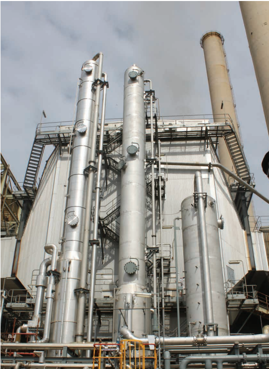
Figure 8: Post-combustion CO 2 capture plant
