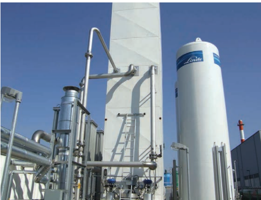
Figure 9: Air separation unit.
